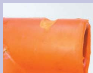
Physical Damage: Rope burns, deep cuts and punctures are cause for rejection.
